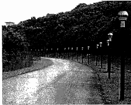
Passive vents installed at Taman Beringin Safe Landfill Restoration project in Kuala Lumpur
